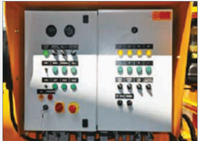
Simple, straightforward control panel
